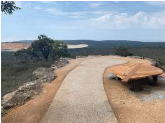
Above: Under construction - the new lookout on Alcoa Boundary track will be part of the Anglesea Heath Bushwalking Trail.
